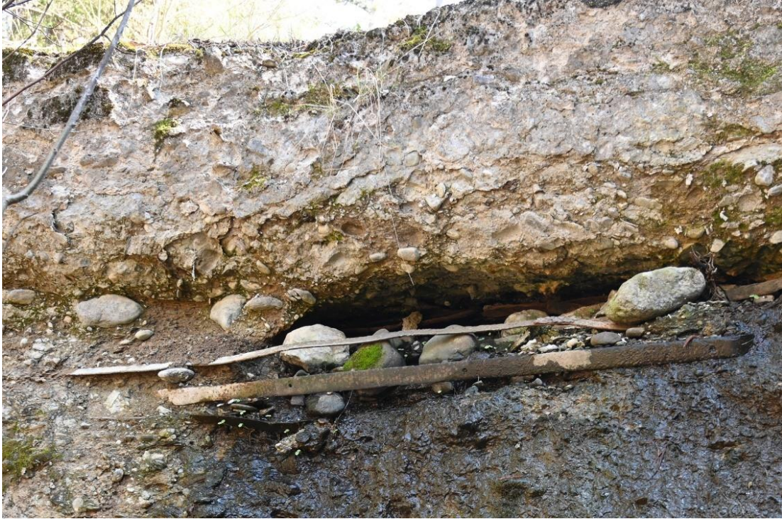
Figure 55. View of exposed metal reinforcement elements on the left side downstream face of structure; also note the concrete aggregate sizes and volume.
