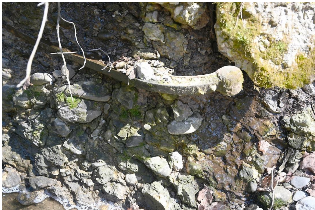
Figure 56. View of an exposed metal reinforcement element embedded in the right apron wall.
