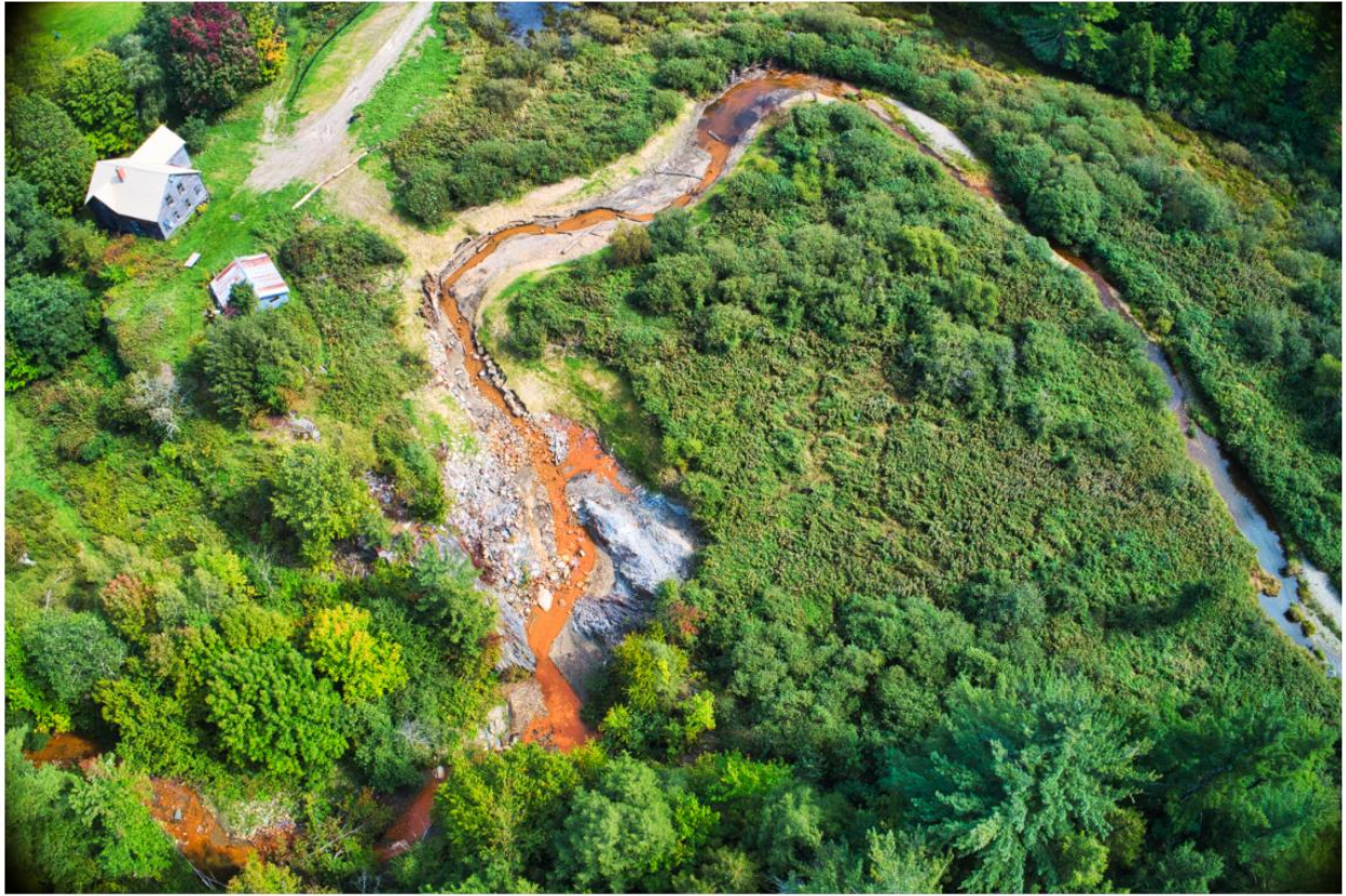
Aerial Photo of the Bogue Branch in the area of the removal of Johnsons Mill Dam. Credit Dana Allen of FluidState Consulting - September 21, 2021.
